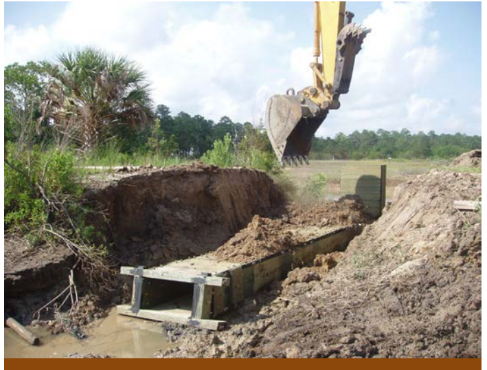
Installation of rice trunk for water level management. Joe Cockrell, USFWS
