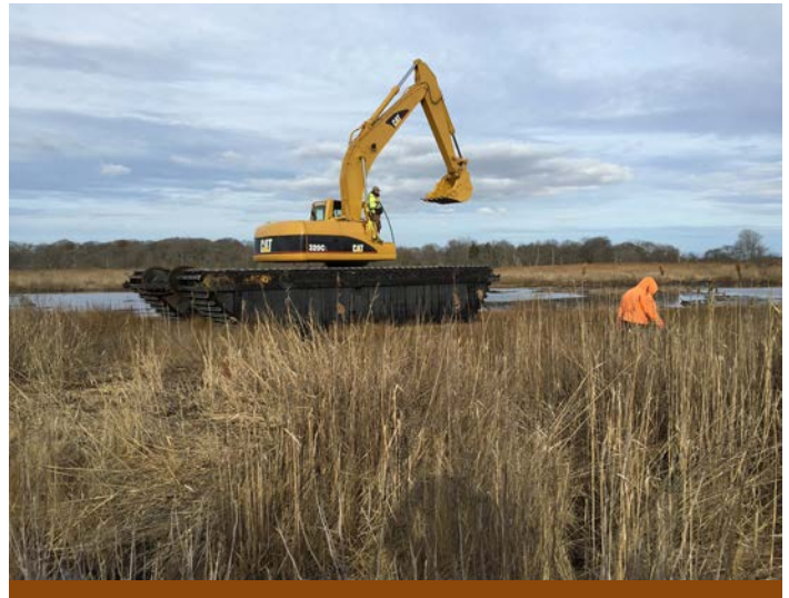
A low ground pressure excavator is moved into position on the salt marsh at Seatuck National Wildlife Refuge to spread freshly dredged sand in waterlogged section of marsh. C. Comber, USFWS
